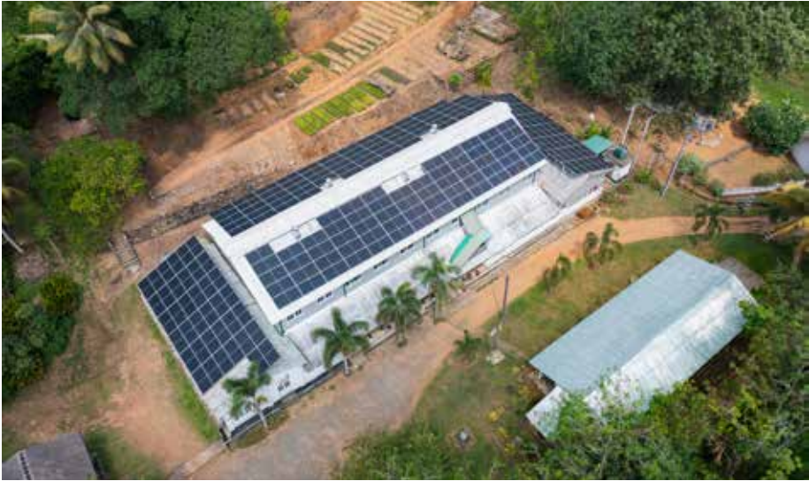
Factory rooftop solar installed at Kobowela
