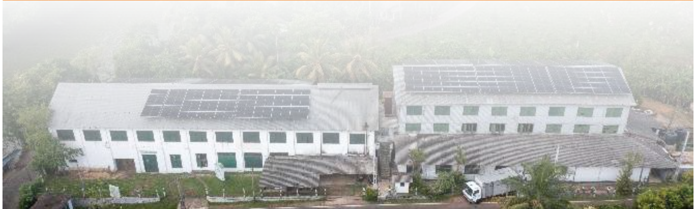
Neuchatel Rubber Processing Center Rooftop Solar System
