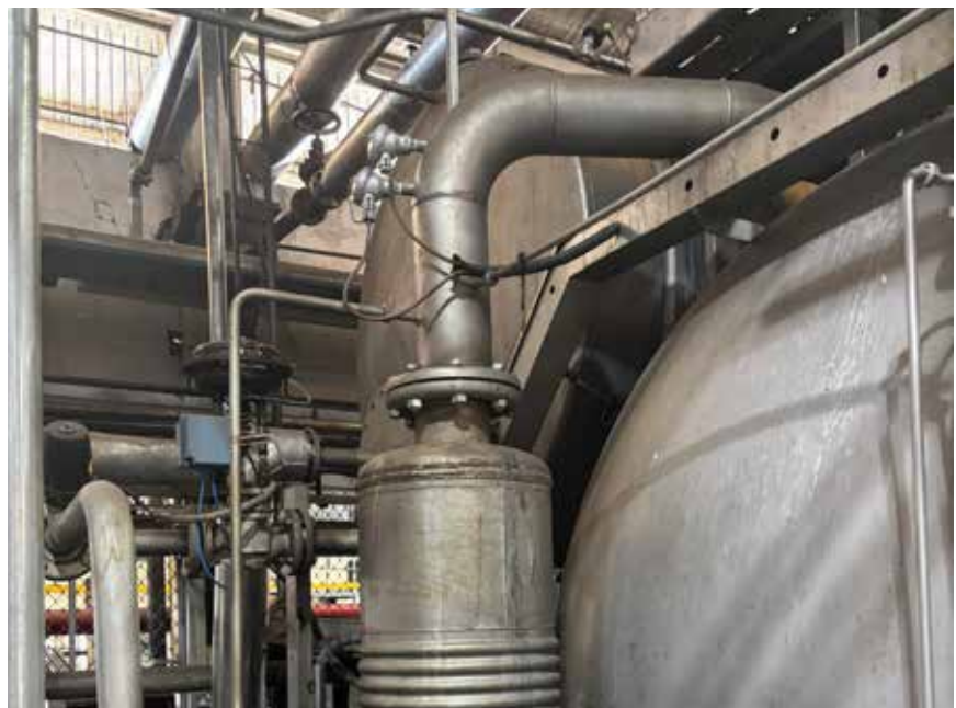
Condensate Water Recovery Project
