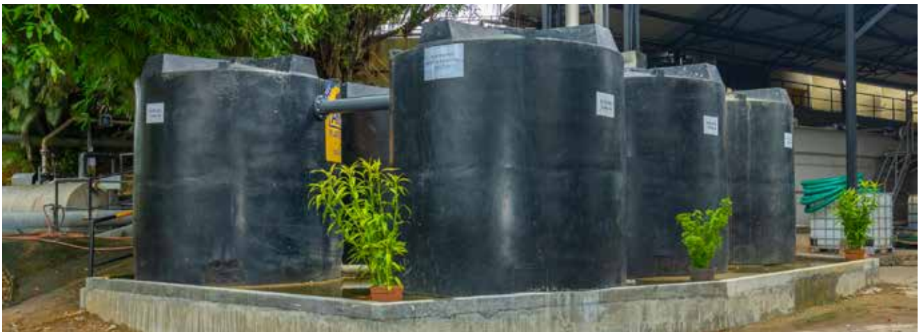
Blow down water recovery system
