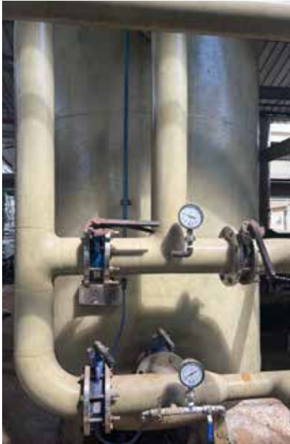
Water treatment optimization of Sand Filtration
